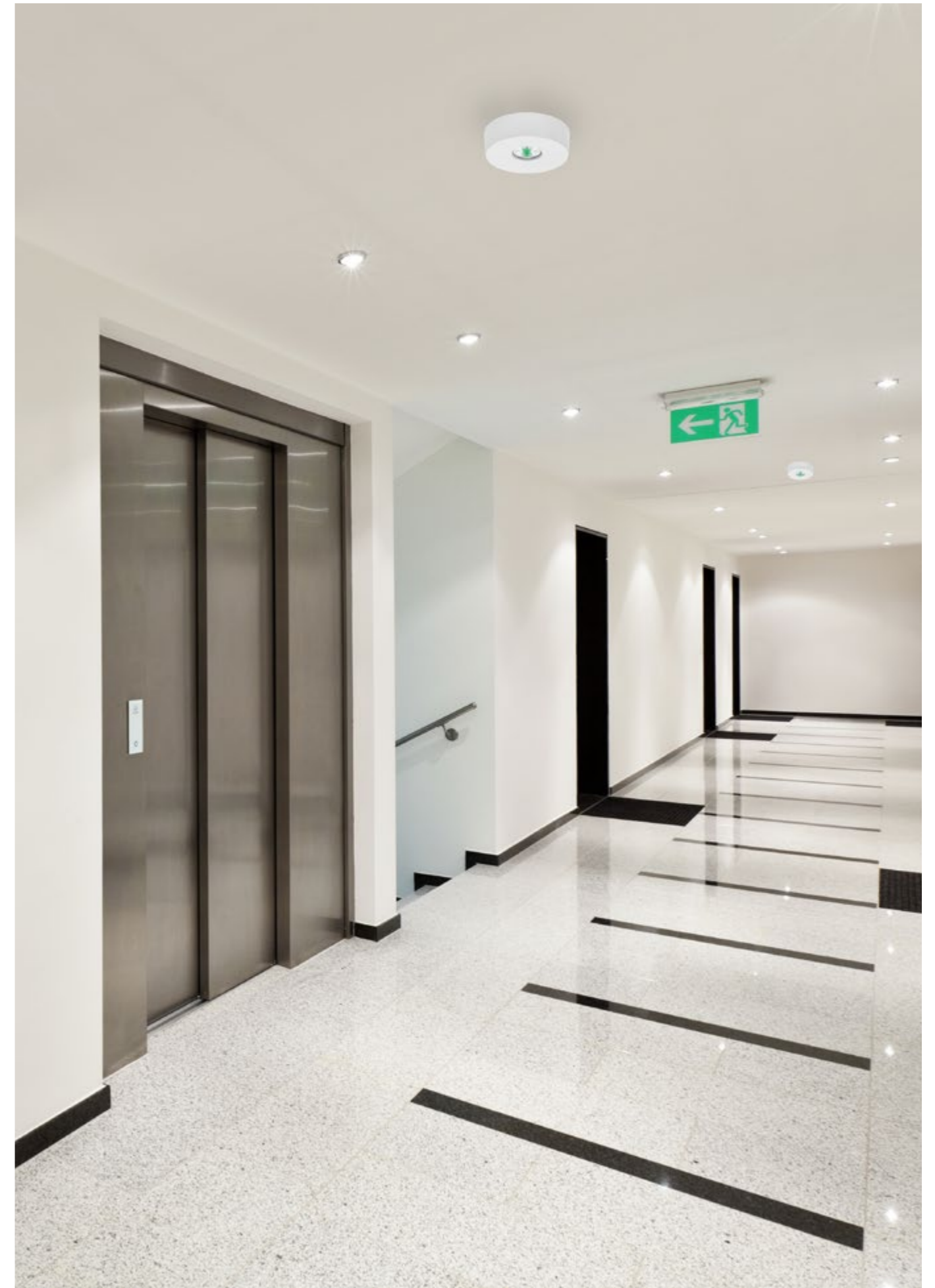
Application of Dot LED CS - corridor in an apartment building.
